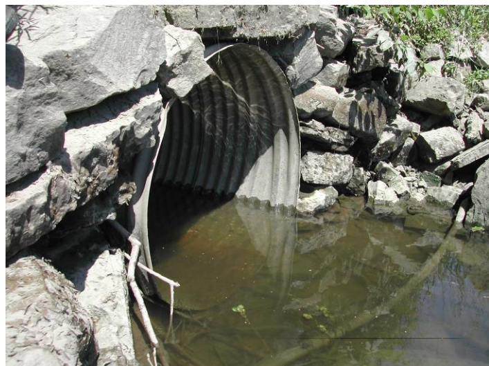
Culverts are used to pass streams and tributaries under roads or other developed properties. If not properly designed and installed, they can disrupt fish and wildlife movement and wash out during floods. (Photo: Carl Alderson, NOAA)
