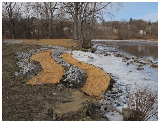
An “ecologically enhanced, engineered shoreline” was built in Coxsackie, NY. The shore included a series of terraces made of stone and plantings. The shoreline was designed to protect a public parking lot while enhancing shoreline and river habitats.
